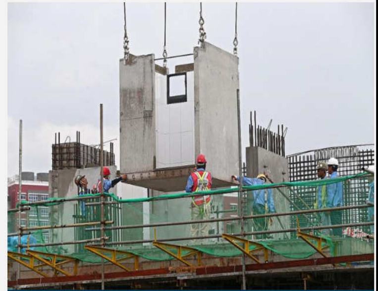
Prefabricated bathrooms units are assembled with finishes in a factory before it is transported to a construction site for installation.
